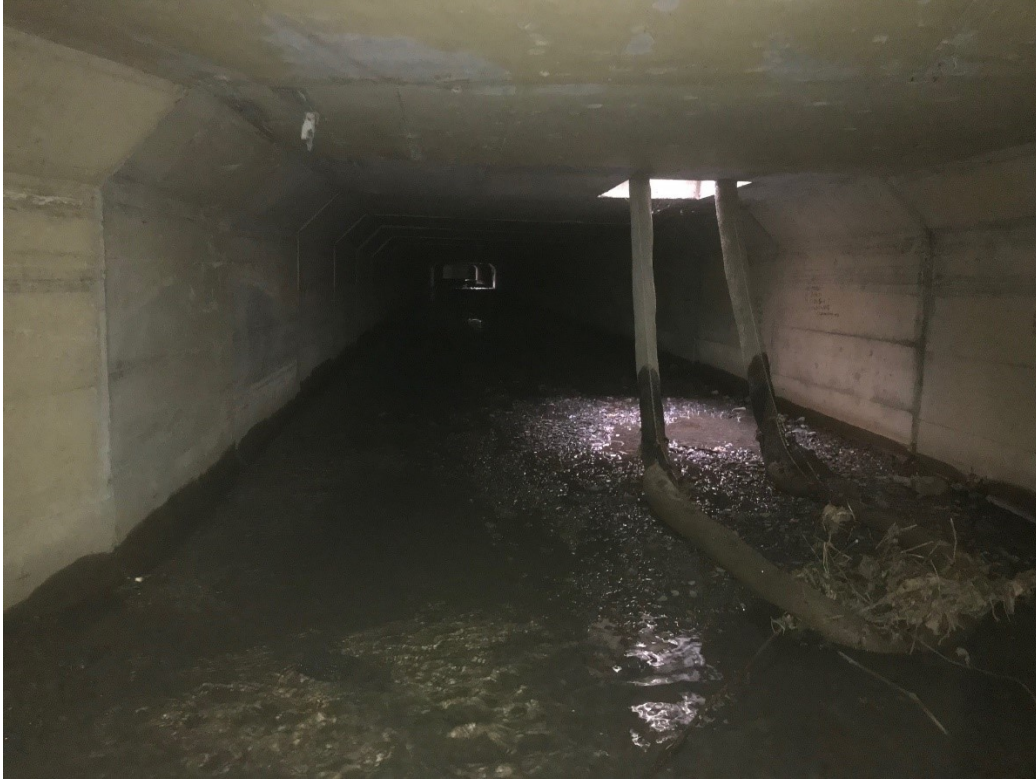
View upstream towards Main Street under Clauverwie Road showing minor aggradation
