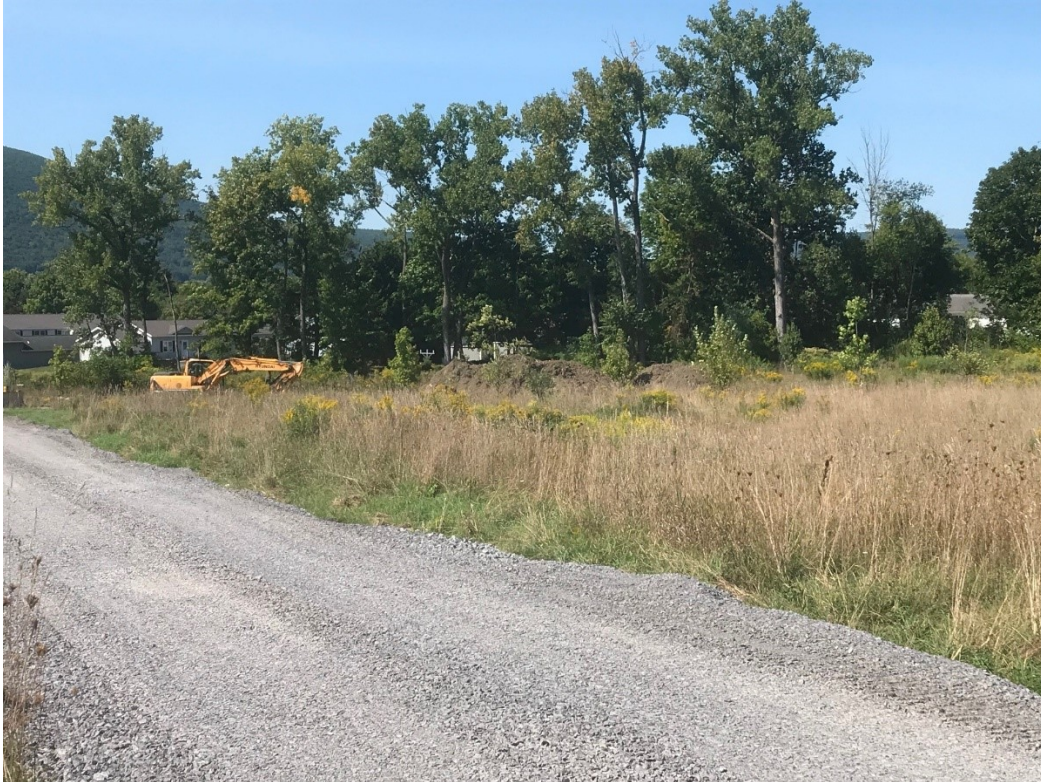
Spoils pile from cleanout 9/5/2024
