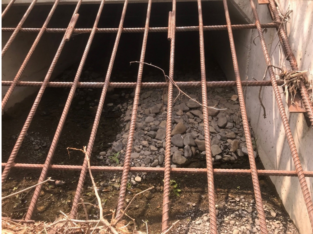
View into new culvert inlet showing some larger deposition for approximately 20 feet into conveyance
