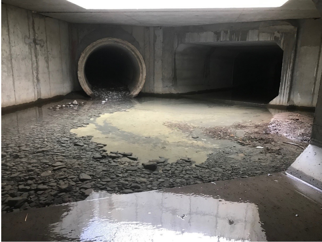
Inside lower cleanout chamber at convergence of old and new primary culverts
